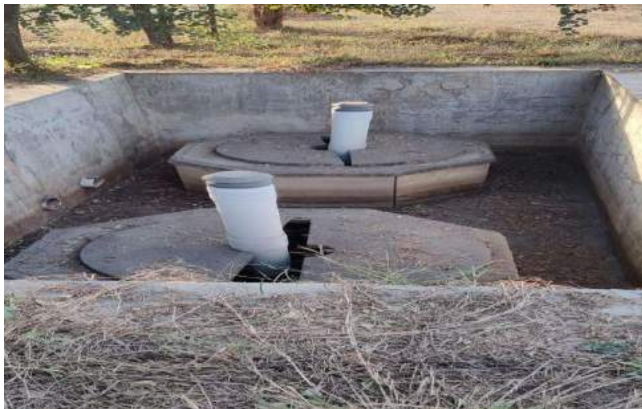
Fig 7.1: Rain water Harvesting in the plant premises
