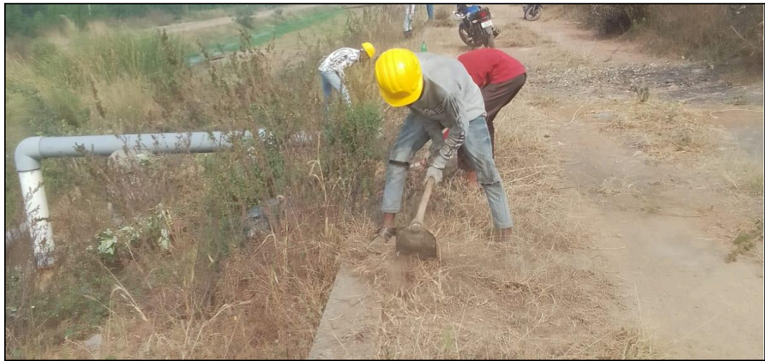
Figure 19: U/S Side Brick lining and Dowel bank. Size - depth 200 mm and wide 100 mm.
